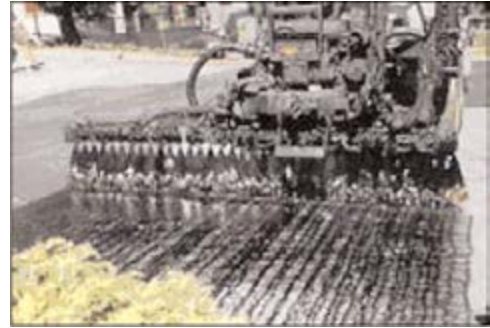
Close-up of unacceptable streaks of asphalt tack coat (refer to Part II C of this brochure).
